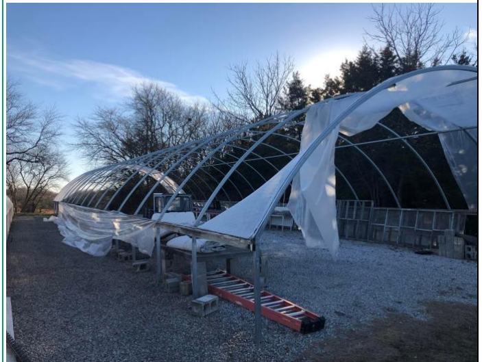
High Tunnel Damage—Johnson County
